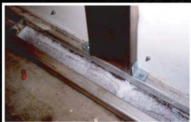
Actual photograph of a competitor's welded aluminum dasherboard frame. Broken weld repaired (by others) by mechanically fastening the joint.
